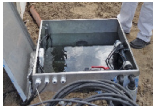
Automated water source
